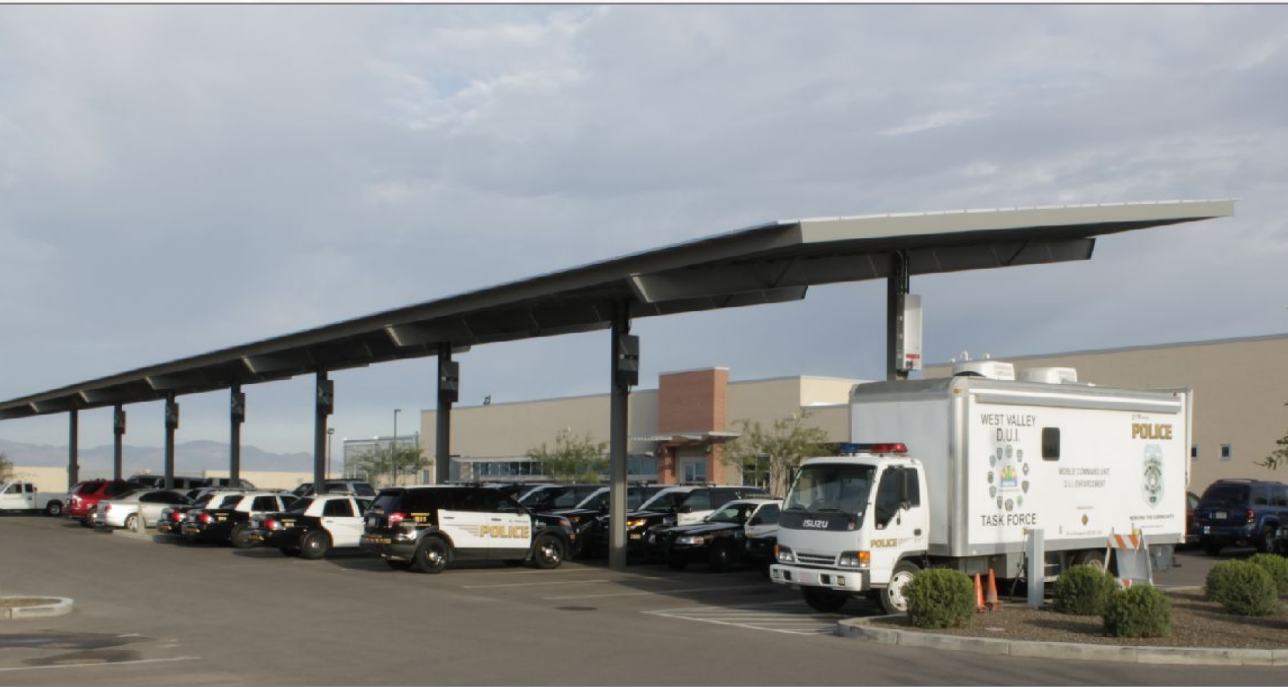
Police Station PV carport array – 131 kW
